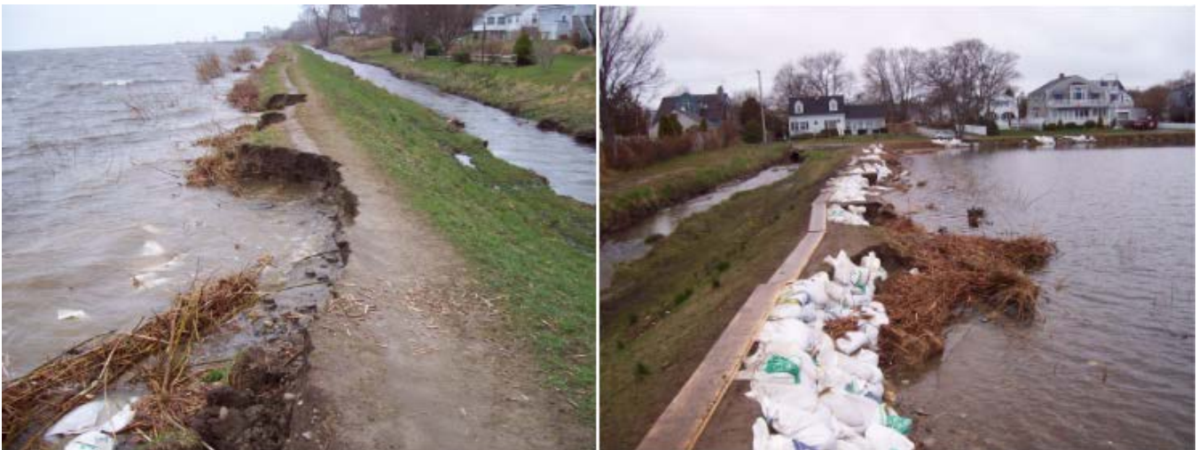
Figure 5: Flood damage at the west embankment of the South Easton Pond Dam after the April 2007 Nor'easter.
