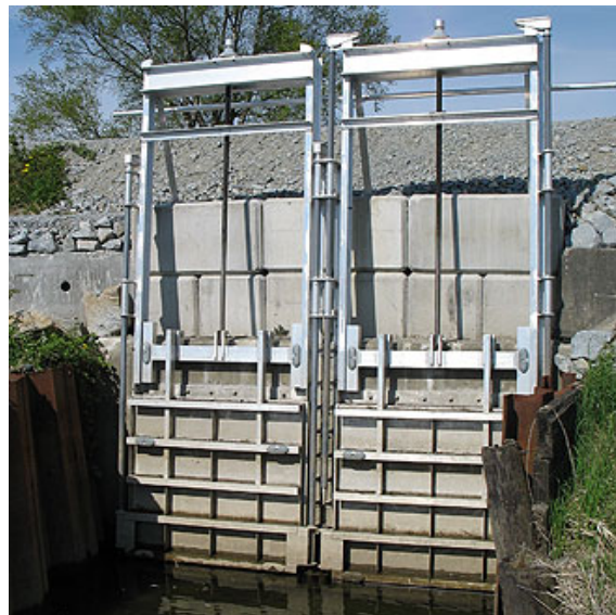
Figure 9: Combination sluice/flap gate.
